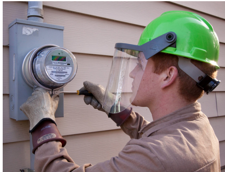
Smart electrical grids have generated a significant fraction of the revenue for the IoT to date. Here, a technician installs a new smart meter at a house in Portland, Oregon, USA.
